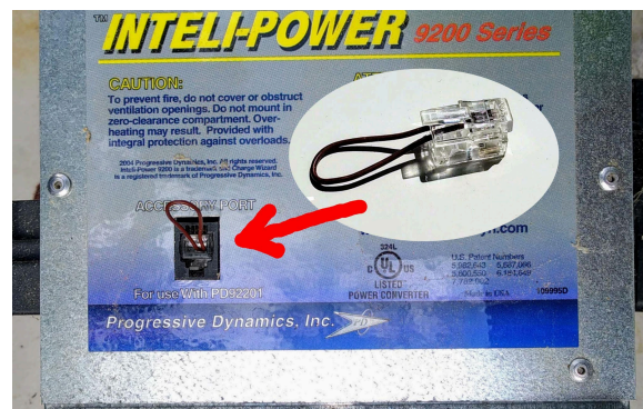
Converter with boost plug installed
